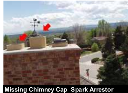
Missing Chimney Cap Spark Arrester
