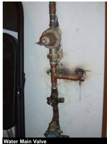
Water Main Valve
