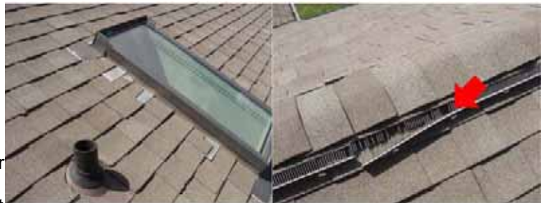
Roof Views, Damaged Ridge Vent
