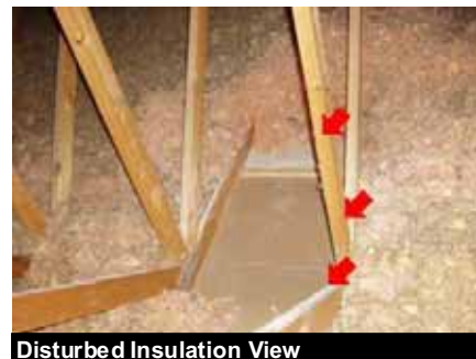
Disturbed Insulation View
