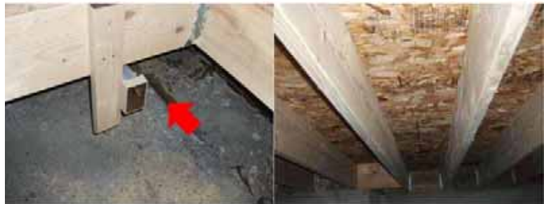
Additional Views, Ventilation System
