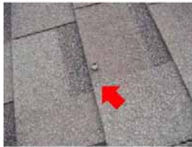
Isolated Roof Issues
