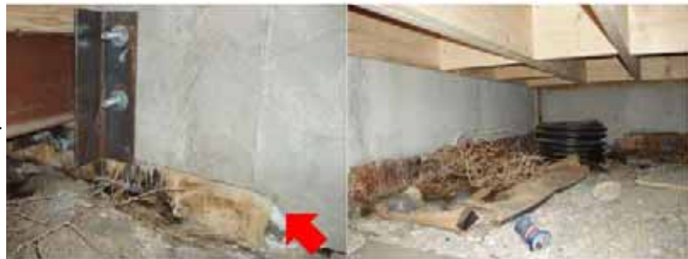
Crawlspace Views, Decaying Cardboard
