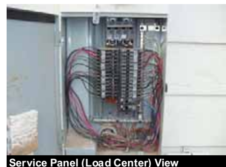
Service Panel (Load Center) View
