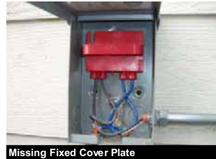
Missing Fixed Cover Plate
