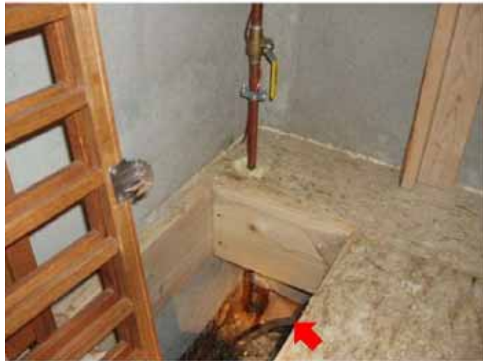
Sump Area and System
