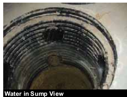
Water in Sump View
