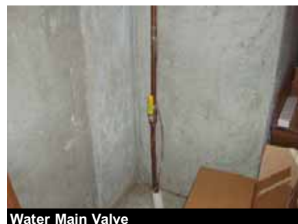
Water Main Valve
