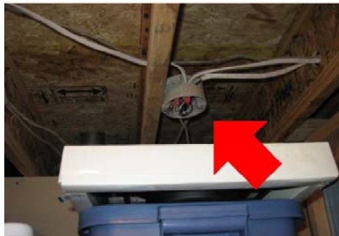
Open Recptacle & Junction Boxes
