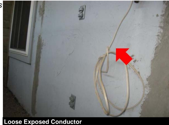
Loose Exposed Conductor
